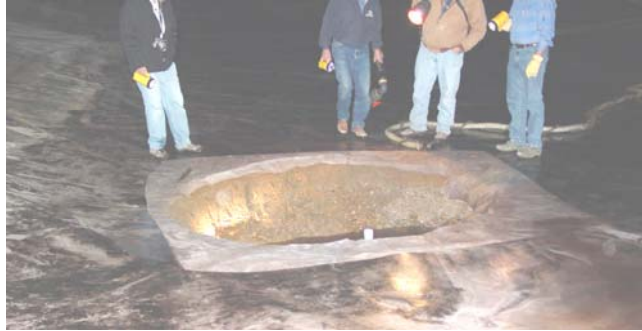
Figure 2. Photo of sinkhole in Case History #1.
