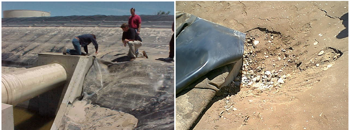
Figure 3. Photos of ripped geomembrane next to penetration, and sinkhole in Case History #2.
